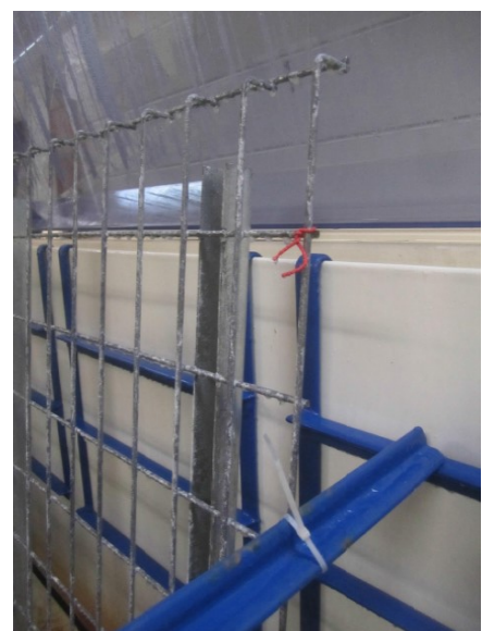
ZINC-COATED DECK (White Rust Visible)
