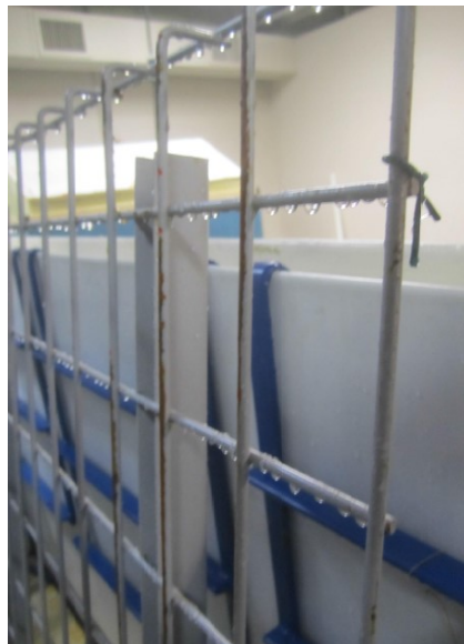
POWDER-COATED DECK (Red Rust Visible)
