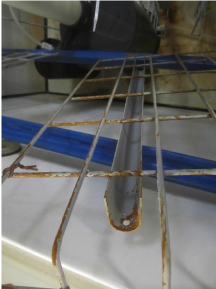
PAINTED DECK (Red Rust Visible)
